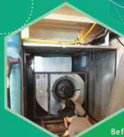
Before Centrifugal blower system
