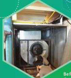
Before Centrifugal blower system
